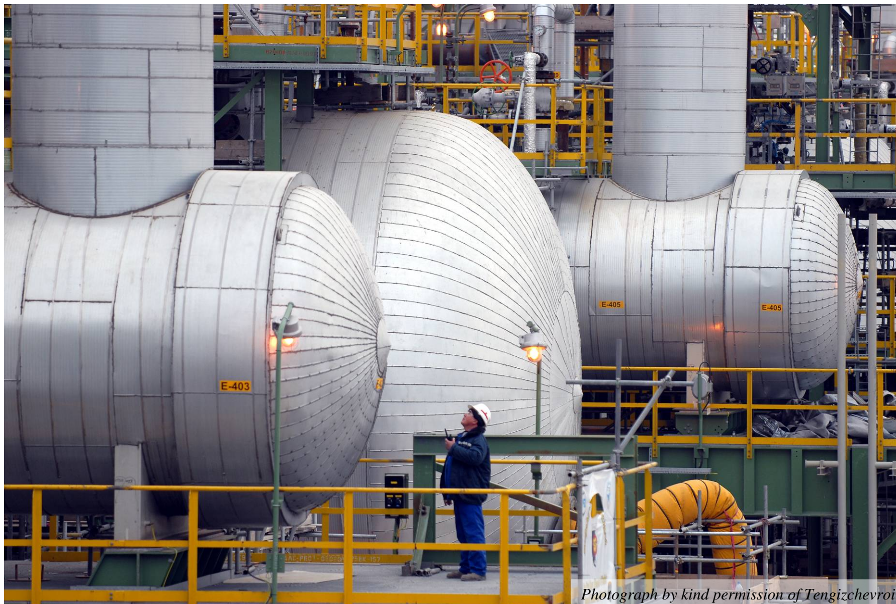
Photo 4: Reheaters and Condenser
